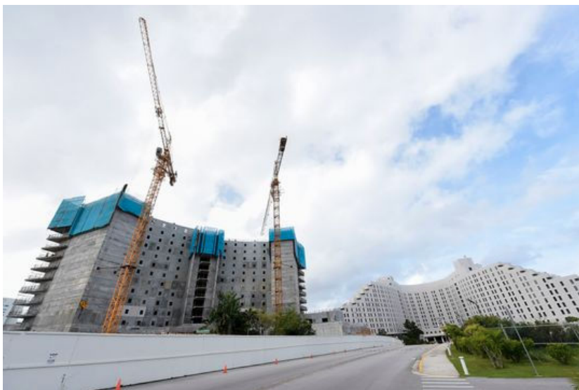
The construction site of the Tsubaki Tower hotel project beside Hotel Nikko Guam in Tumon, Jan. 22, 2019. (Photo: Frank San Nicolas/PDN)
