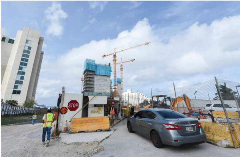
The construction site of the Tsubaki Tower hotel project in Tumon, Jan. 22, 2019. (Photo: Frank San Nicolas/PDN)
