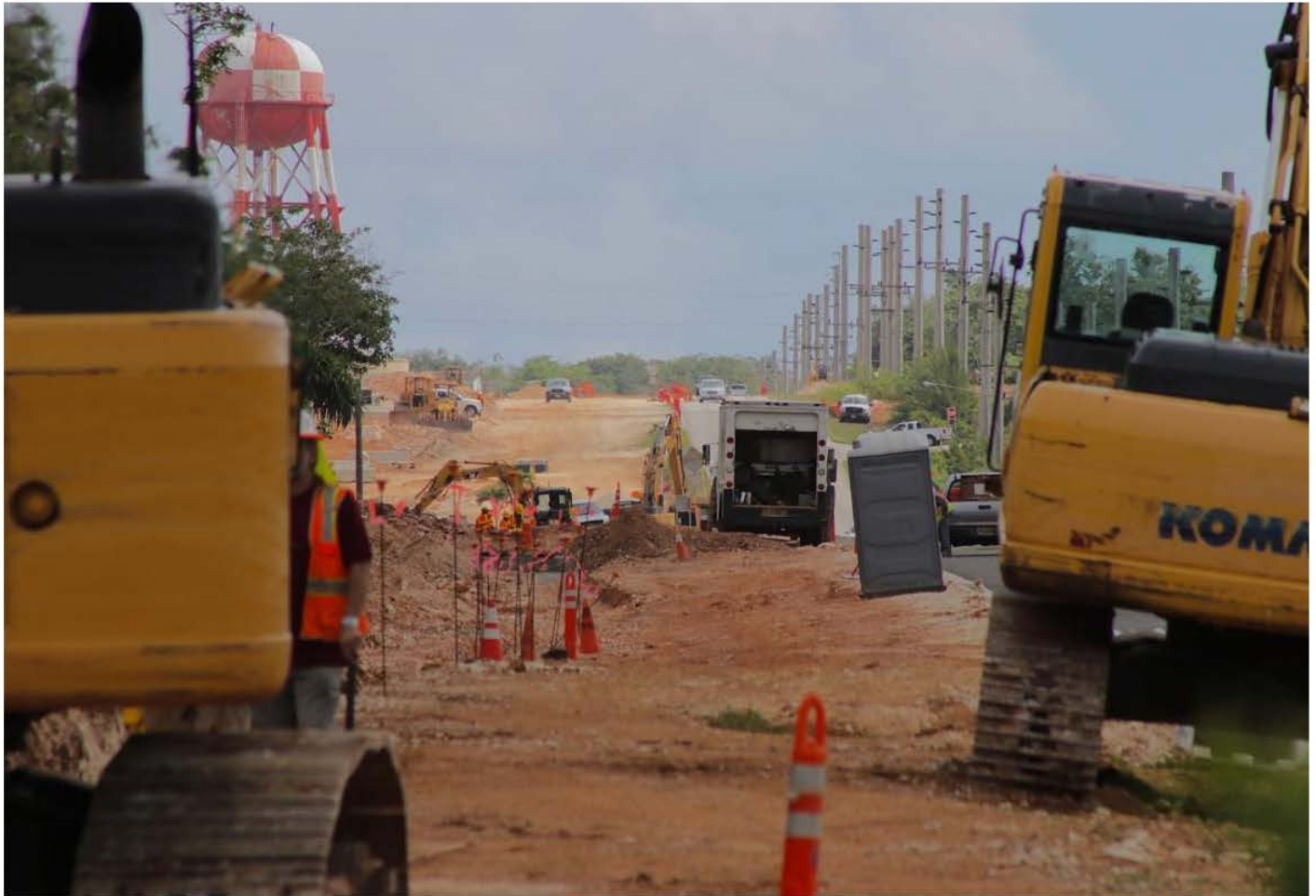
ROUTE 3: Work continues on the road widening project along Route 3 in Dededo in April. Some of the military and civilian construction projects related to the military buildup on Guam need additional imported labor. Dontana Keraskes/The Gua Daily Post
