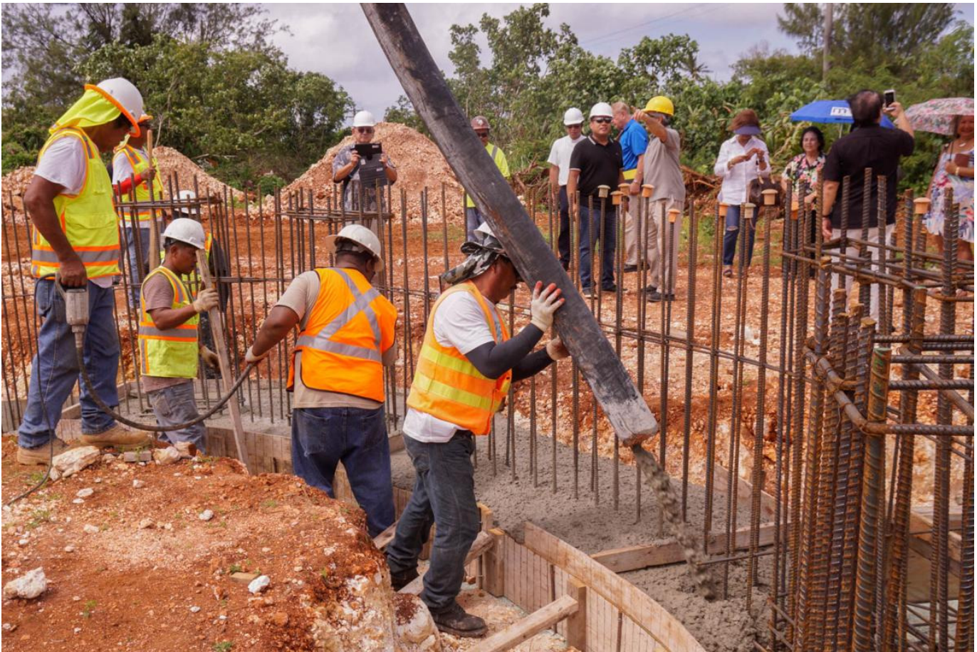
BUILDING: A construction crew works on a project in Dededo. A federal judge has broadened the scope of her decision on hiring foreign workers on H-2B visas. Post file photo
