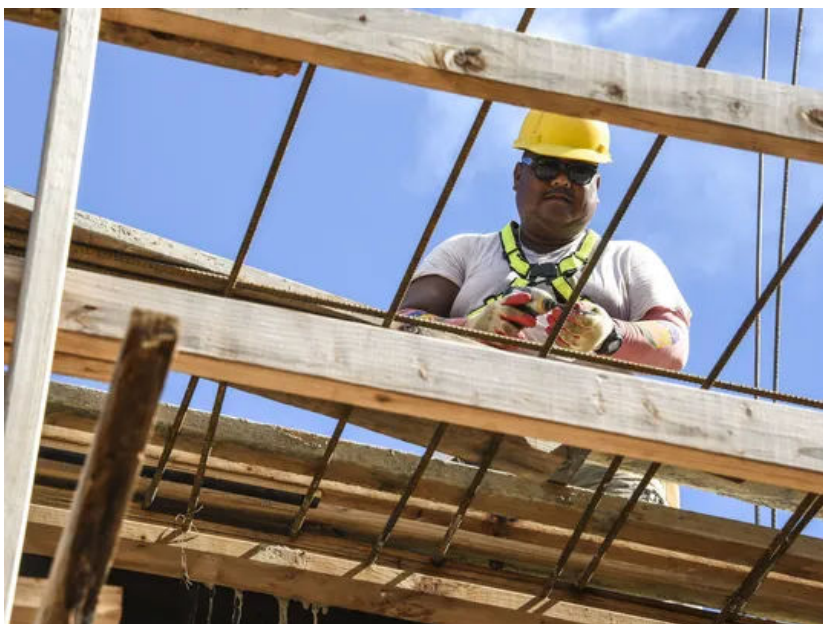
In this Oct. 4, 2016, file photo, carpenter Negs Barrozo prepares to fasten lumber together into a form, as he and other 5M Construction Corporation employees work at a building project in Tamuning. A near 100-percent rejection rate for Guam H-2 worker visa applications has short- and long-term implications for the island's construction industry. Carpenter Negs Barrozo prepares to fasten lumber together into a form, as he and other 5M Construction Corporation employees, work at a building project in Tamuning on Tuesday, Oct. 4. 5M is one of a dozen Guam businesses that sued the federal government over worker visas. (Photo: Pacific Marketplace file photo)
