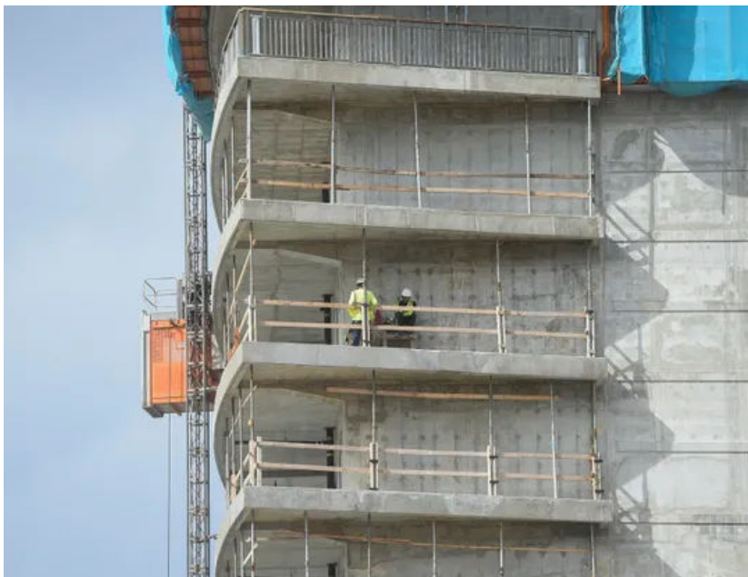
Construction workers on the site of the Tsubaki Tower hotel project in Tumon, Jan. 22, 2019. (Photo: Frank San Nicolas/PDN)
