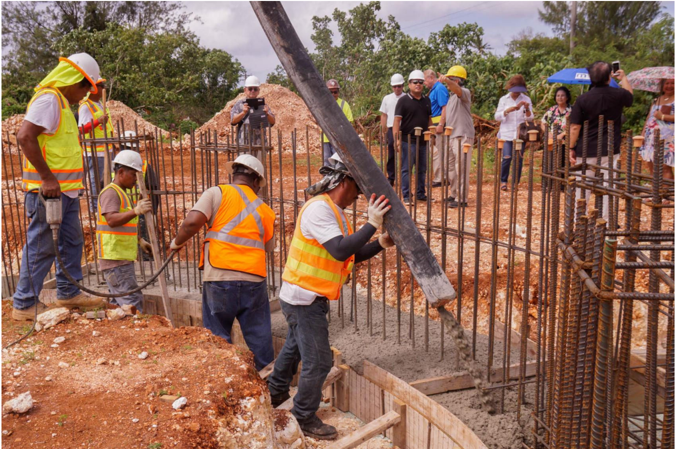
MEN AT WORK: A construction crew works on a project in Dededo. Attorney Jeff Joseph recently filed a motion in the District Court of Guam asking the judge to hold the U.S. Citizenship and Immigration Service in contempt and impose sanctions on the federal agency for its continued denial of H-2B petitions from Guam employers. Post file photo
