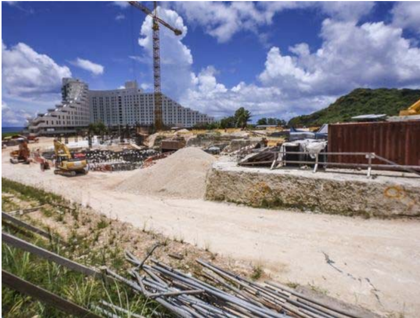
An overview look of the construction site of the Tsubaki Tower, as seen in Tumon, on Wednesday, Aug. 23, 2017. The hotel project, started in March 2016 by Tokyo real estate giant Ken Corp., is slated to reach a height of 26 stories and cost an estimated $150 million to build, according to Pacific Daily News files. Subcontractor 5M Construction said manpower issues have delayed work on the project. (Photo: Rick Cruz/PDN)
