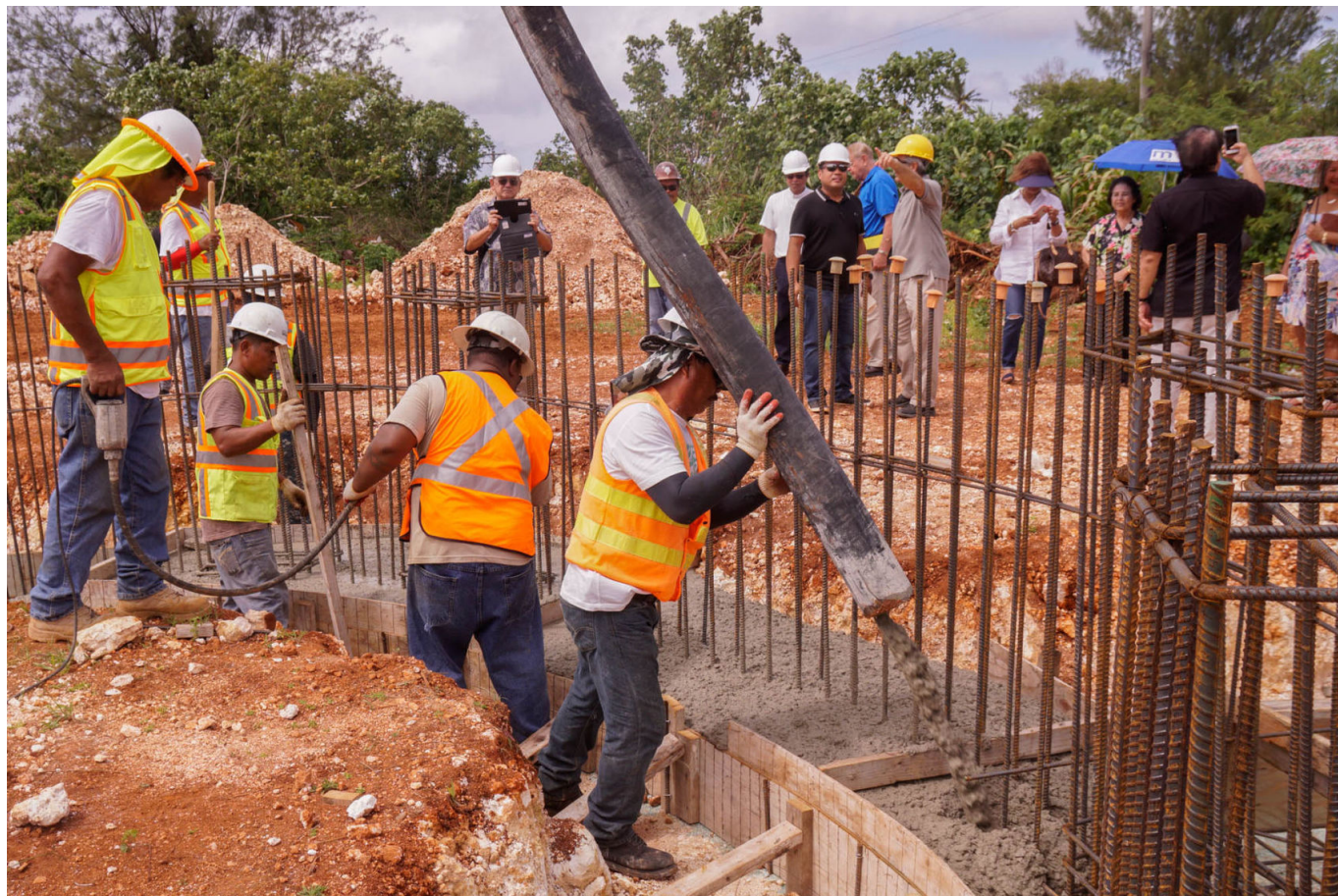
CONSTRUCTION: A construction crew works on a project in Dededo. Post file photo
